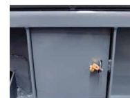
Drainage safety valve at the bottom of the fuel tank
