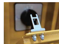
The panel of the voltage switch provides protection function, the engine will stop upon opening of the panel
