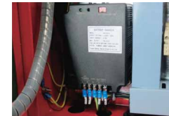
Battery Charger Enables the battery to be in constant recharging in which the generator set can be started at all time
